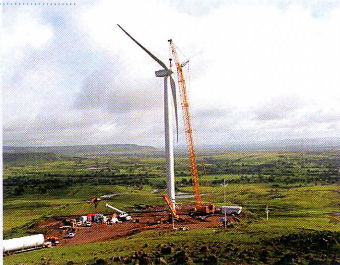
Kenersys is equipping an 8 MW wind farm in Maharashtra, India's second largest wind state after Tamil Nadu.
